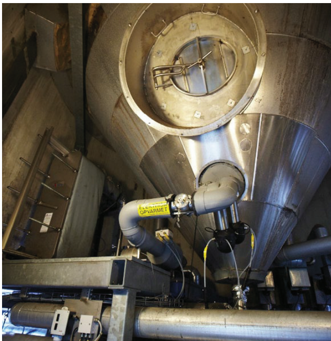
The Iso-Mix system installed in Carlsberg's fermentation tanks include a plate type heat exchanger, which enables much faster cooling.
